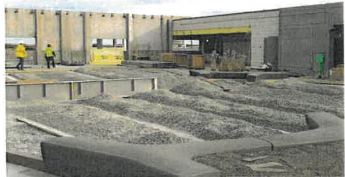
The rooftop plaza will include a central green, roof garden, seating, canopies and catering facilities
