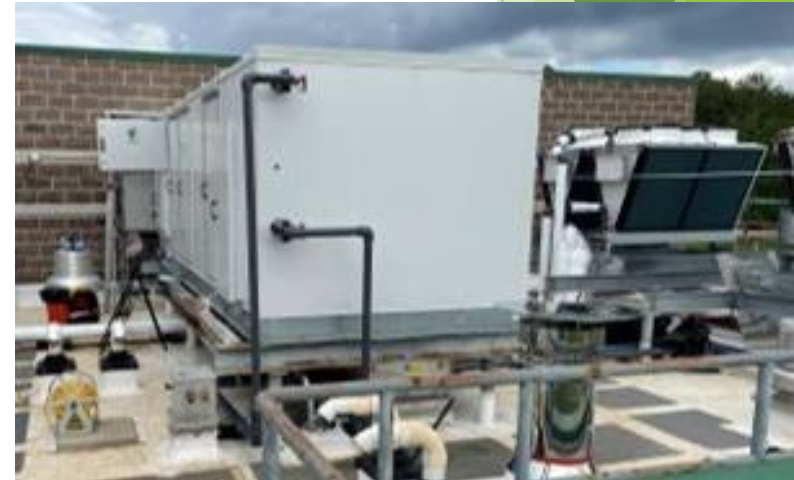
South Run Rec Center Pool Units (top)
