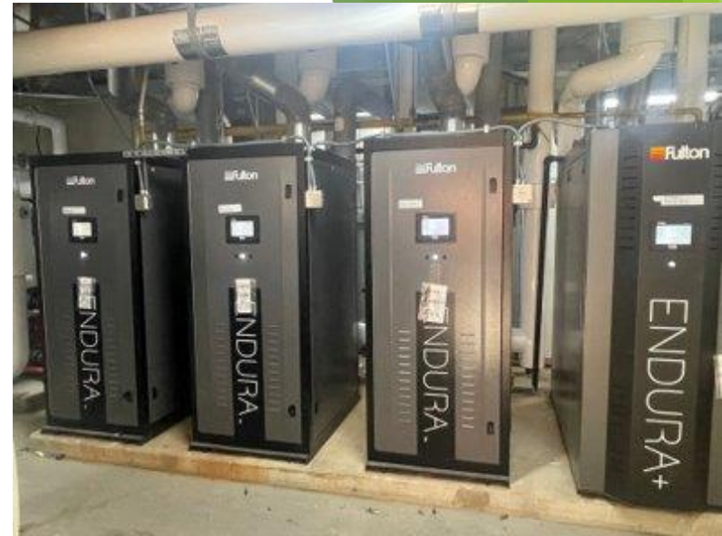
Cub Run Rec Center Boilers (top)
