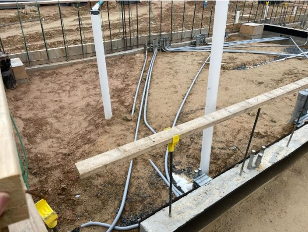
Underground conduits and piping
