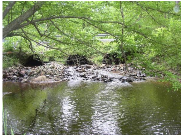
Figure 4-15: Obsolete culvert (Source: KCI)
