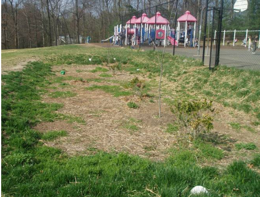
Site photo: Existing bioretention filter in need of amendments.
