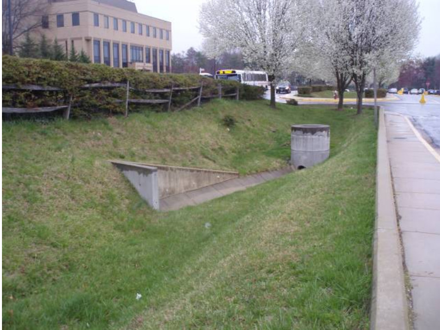
Site photo: Existing dry pond located in a parking island in the site parking lot.
