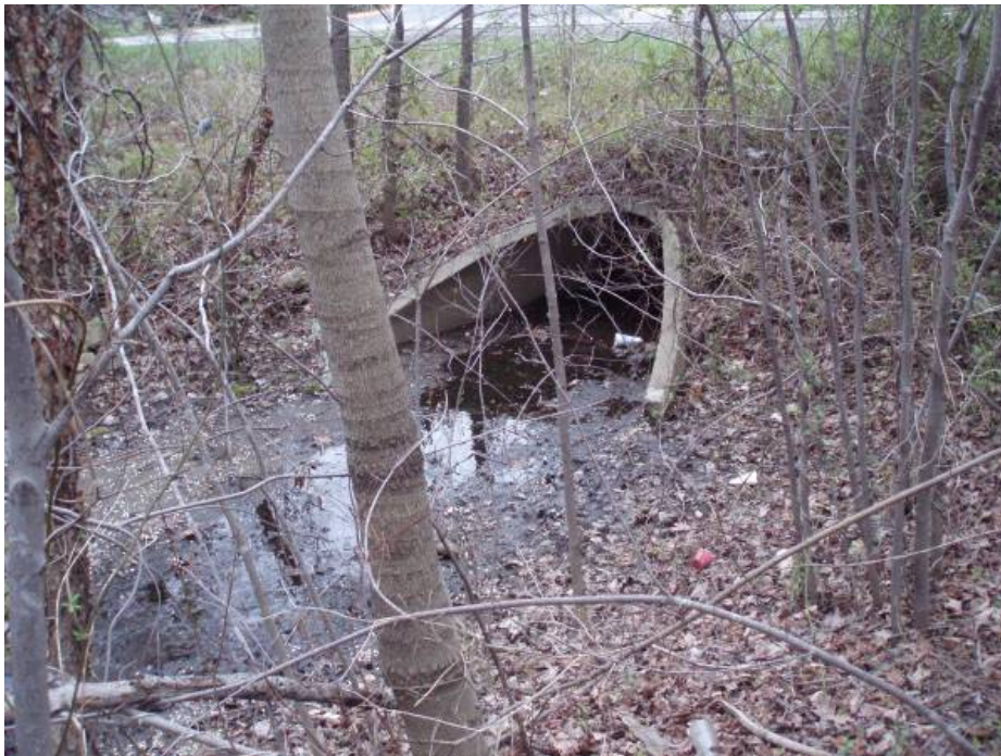
Site photo: Outlet of storm drainage system on east side of Newington Road.
