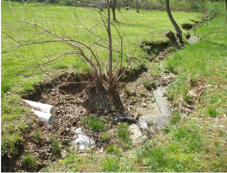
Site photo: Erosion and headcutting caused by roof drains.
