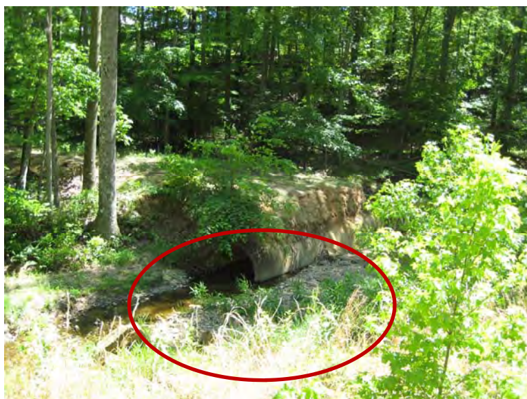
Figure 59: Exposed culvert in Area A
